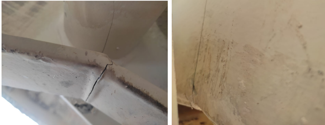
Fig. 2 Fatigue-cracked section of the vibrating feeder
